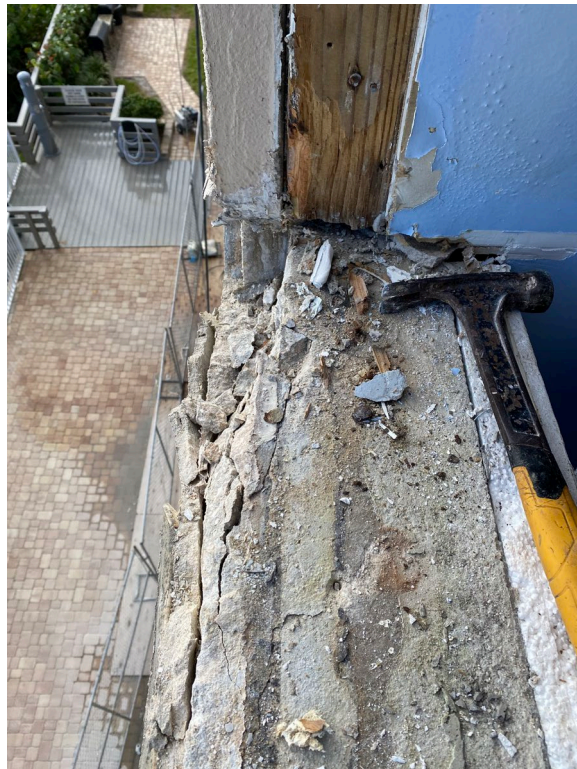
Picture 4: Cracked window sill of Unit 308
